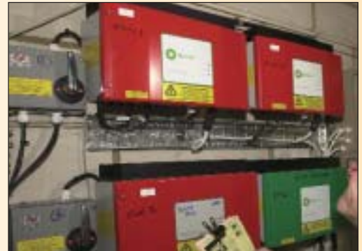
Inverters which convert the DC output from the wind turbine and solar panels into a usable AC power supply
